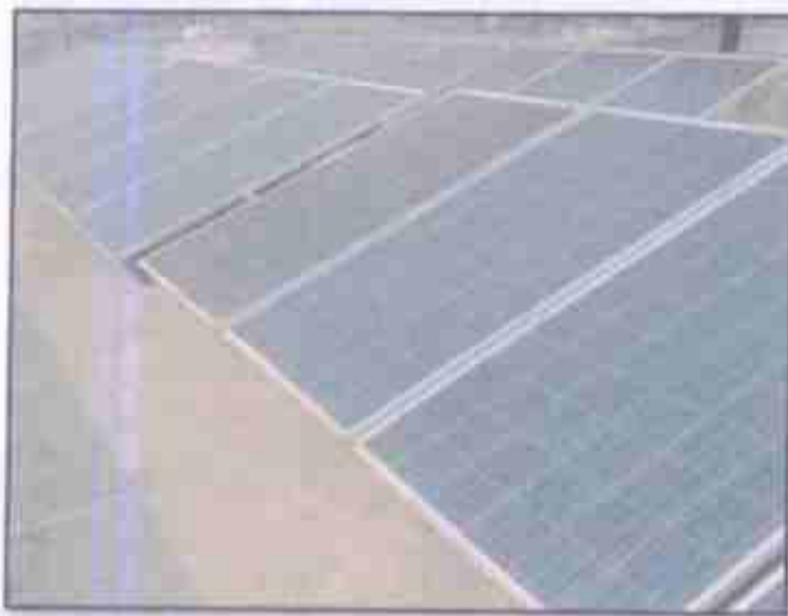
Photograph of Roof Top Solar PV Plant:
