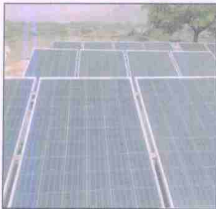
Photograph of Roof Top Solar PV Plant:
