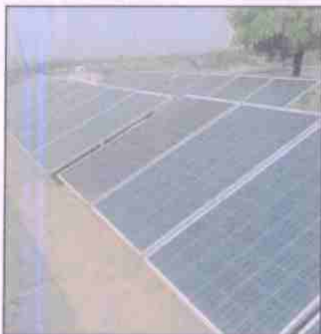
Photograph of Roof Top Solar PV Plant:
