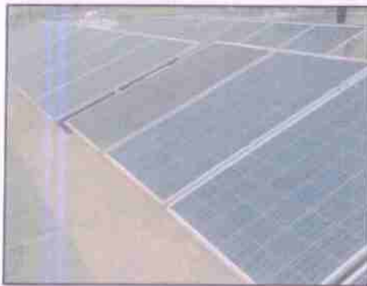
Photograph of Roof Top Solar PV Plant:
