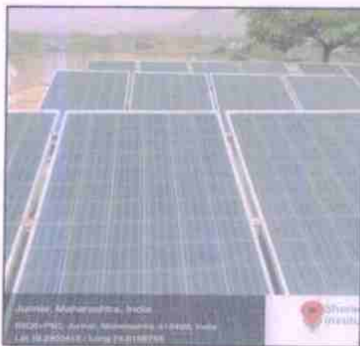
Photograph of Roof Top Solar PV Plant:
