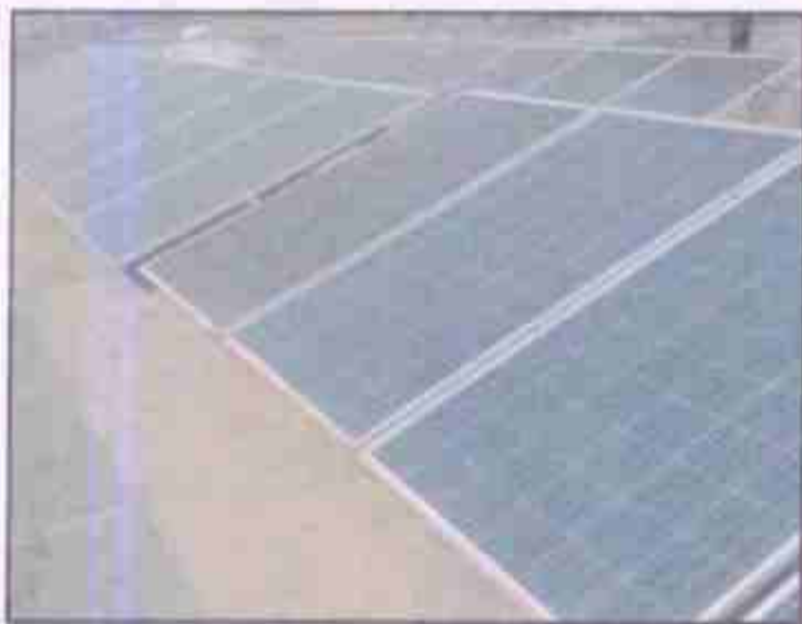
Photograph of Roof Top Solar PV Plant:
