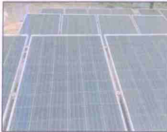
Photograph of Roof Top Solar PV Plant:
